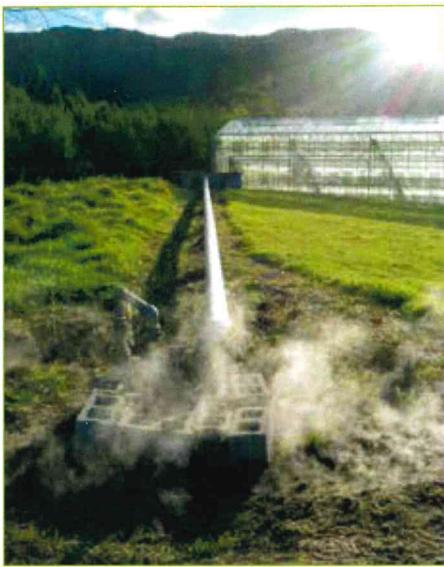
This geothermal bore produces 100°C water that is fed through a heat exchanger, heating water circulated in an internal closed heating system.
