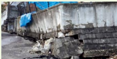
Sendai City (collapsed retaining wall)
