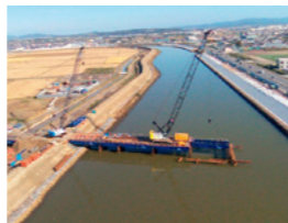
Photo: Construction of a temporary bridge linking piers on the Jokawa River (Higashimatsushima City)
