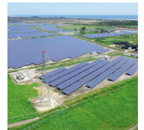
Photo: Mega solar power plant (Iwanuma City)
